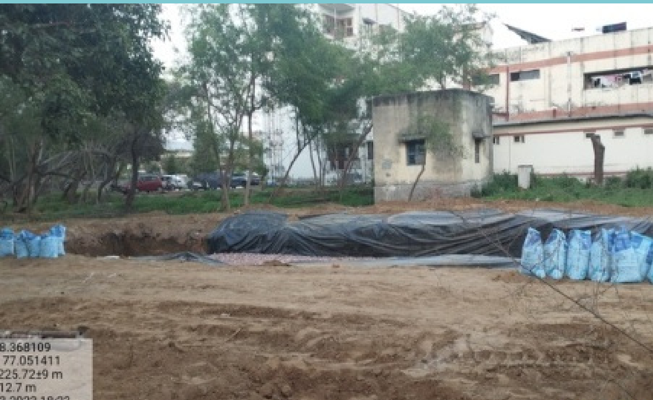
50 KLD TREATMENT SYSTEM
