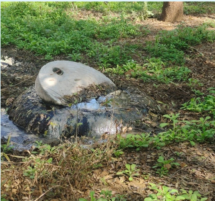
Figure: Sewage Overflow from Manhole
