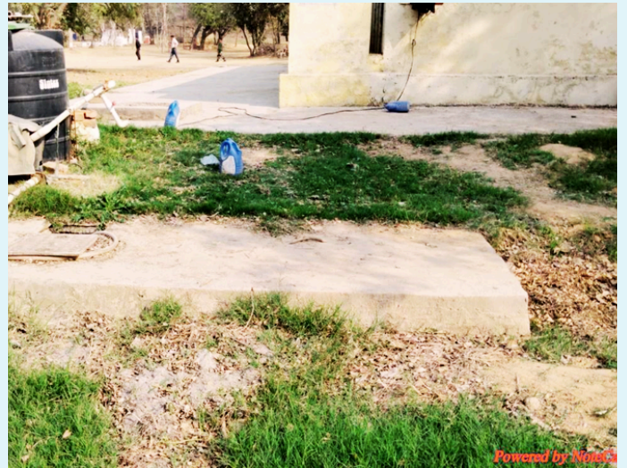
Figure: Septic tanks were leaking and overflowing
