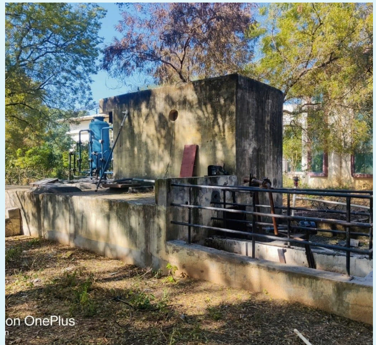
Figure: Defunct Sewage Treatment Plant
