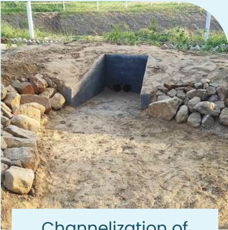
Channelization of Rainwater to the Pond
